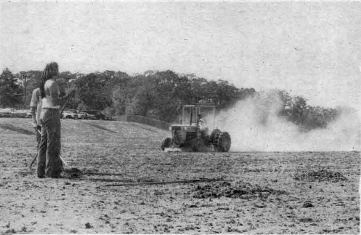
BREAK IT UP: Physical plant workers breaking up the upper athletic field, as a part of a series of treatments to recondition the field. [Photo by Romondo Davis].
